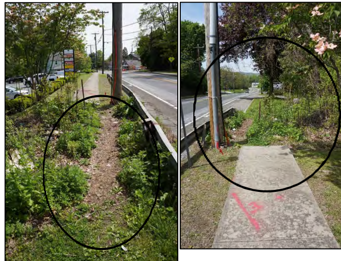
Figures 21 and 22: Sidewalks are essential for pedestrians and worn "goat" paths demonstrate the need for them where they are absent.
